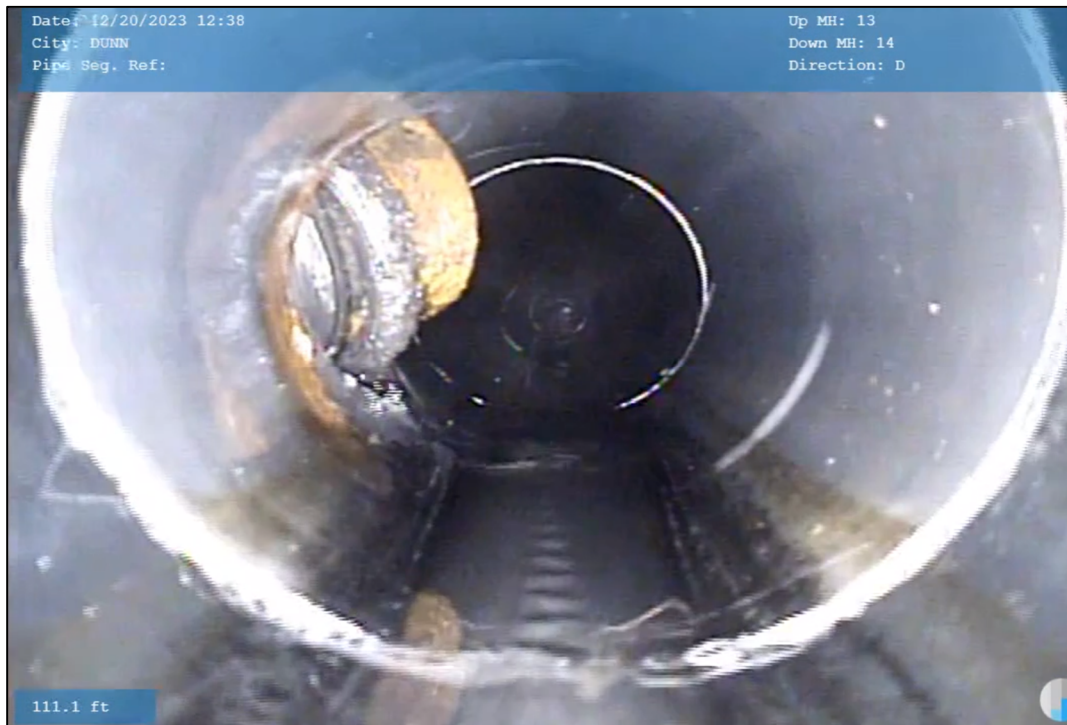
Figure 6: Defective lateral with broken/intruding tap and infiltration. Upstream Manhole: 13, Downstream Manhole: 14 Address: 3054 Shaw Ct.
