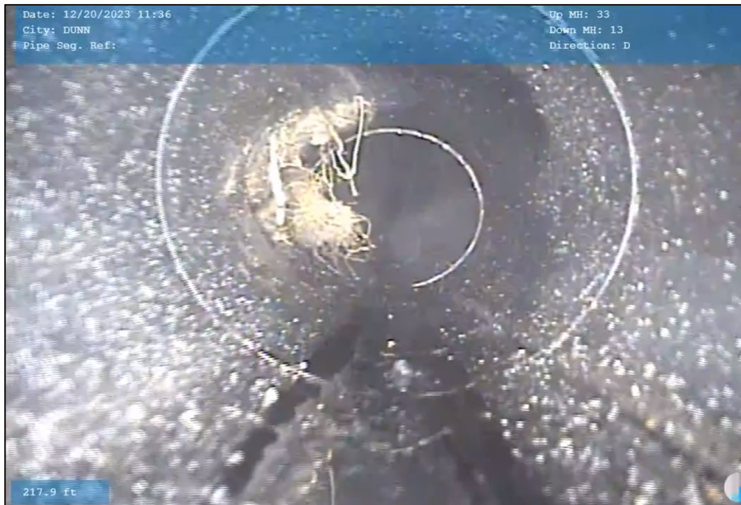
Figure 8: Defective lateral with root blockage. Upstream Manhole: 33, Downstream Manhole: 13 Address: 3036 Waubesa Ave.
