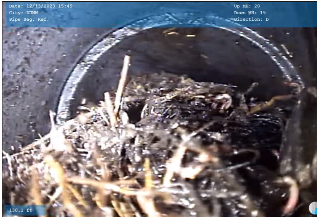
Figure 3: Defective lateral with root blockage. Upstream Manhole: 20, Downstream Manhole: 19 Address: 3094 Waucheeta Trail
