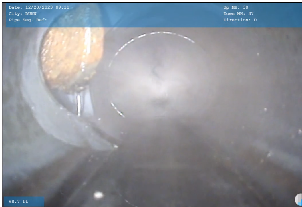
Figure 10: Defective lateral with intruding tap and possible infiltration. Upstream Manhole: 38, Downstream Manhole: 37 Address: 3004 Waubesa Ave.
