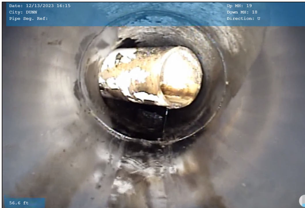
Figure 4: Lateral with tap intruding into sanitary sewer main. Upstream Manhole: 19, Downstream Manhole: 18 Address: 4338 McConnell St.
