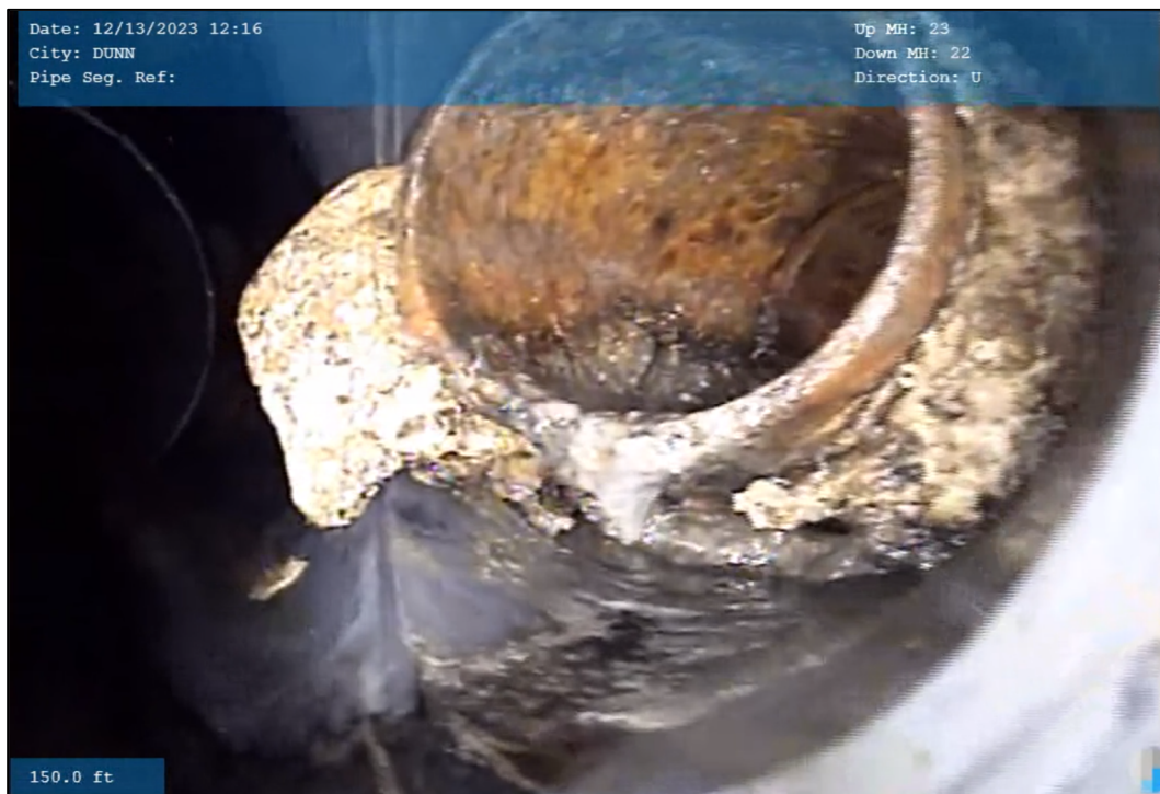
Figure 2: Defective lateral with corrosion and deposits. Upstream Manhole: 23, Downstream Manhole: 22 Address: 3140 Waucheeta Trail
