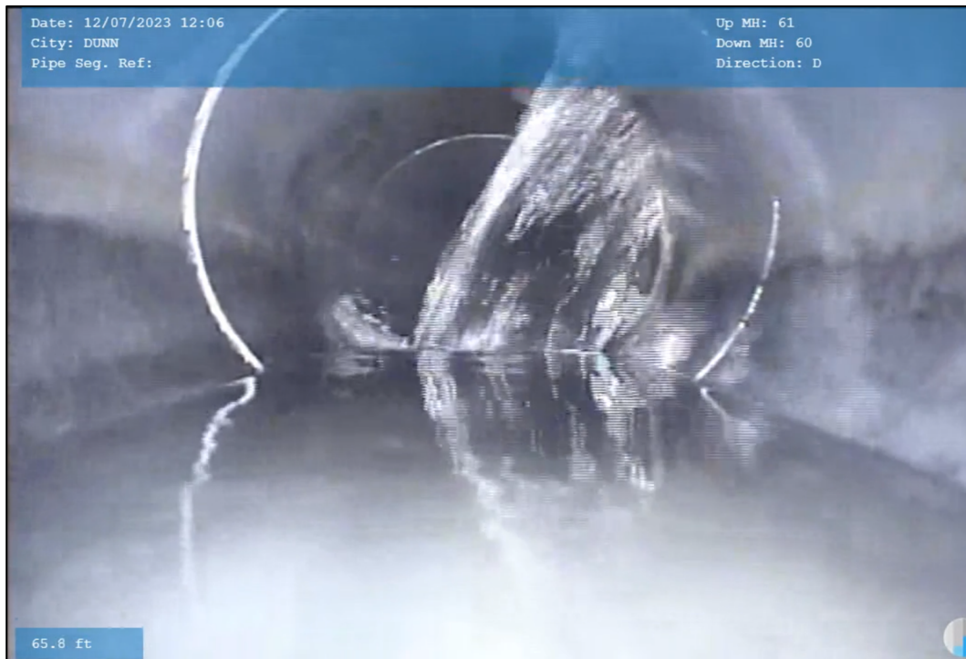
Figure 20: Possible lateral break with significant inflow/infiltration. Upstream Manhole: 61, Downstream Manhole: 60 Address: 2894 Waubesa Ave.
