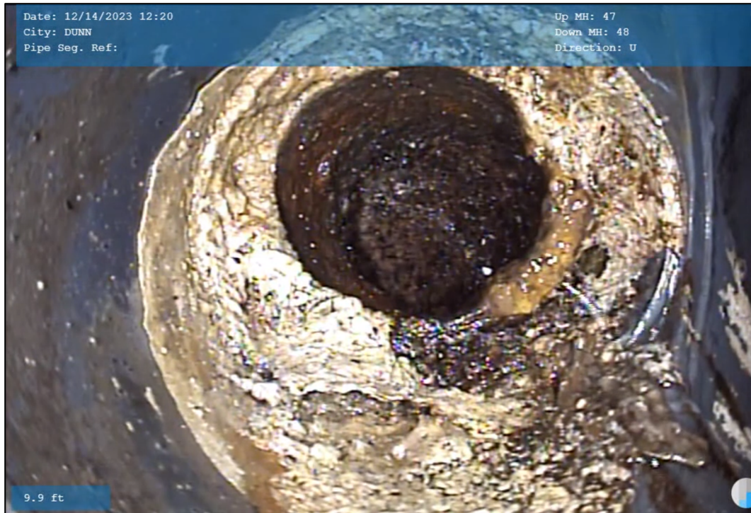
Figure 17: Defective lateral with corrosion and deposits. Upstream Manhole: 47, Downstream Manhole: 48 Address: 2960 Waubesa Ave.
